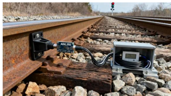
Figure 6: Installation position of the ADXL345 vibration acceleration sensor.
